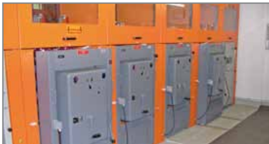
HS- Anlage alt
